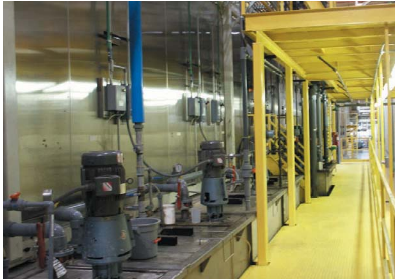
11-Stage Zinc Phosphate Pretreatment System
